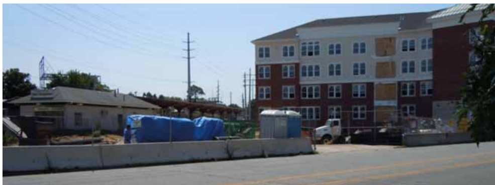
Redevelopment of the West Hempstead Courtesy Hotel site with LIRR station at left
